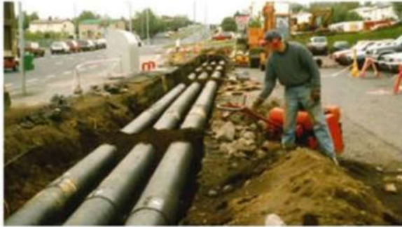
Figure 4. Installment of the Geothermal District heating piping in Iceland, source: www.verkis.is presentation by T. Johannesson, Cornell 2016, used by courtesy of the presenter
